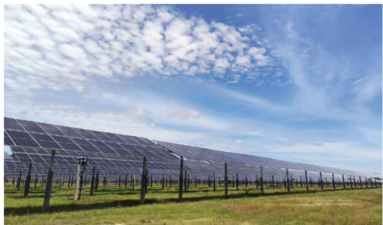
Visual 02: Coara Marang's solar site in Terengganu
