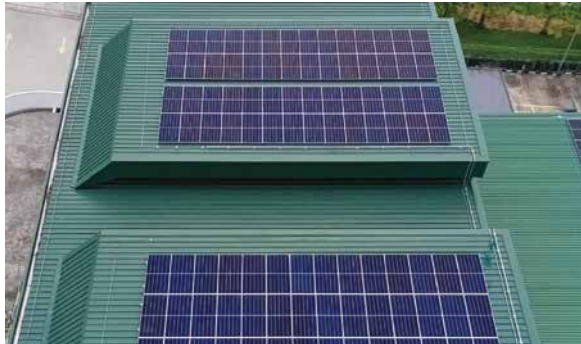
Visual 03: Outspan Malaysia Sdn. Bhd.'s solar roof in Johor
