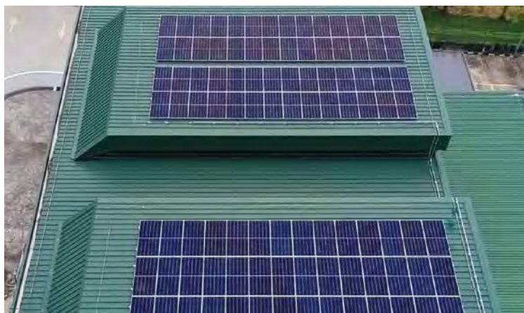
Visual 02: Outspan Malaysia Sdn. Bhd.'s solar roof in Johor
