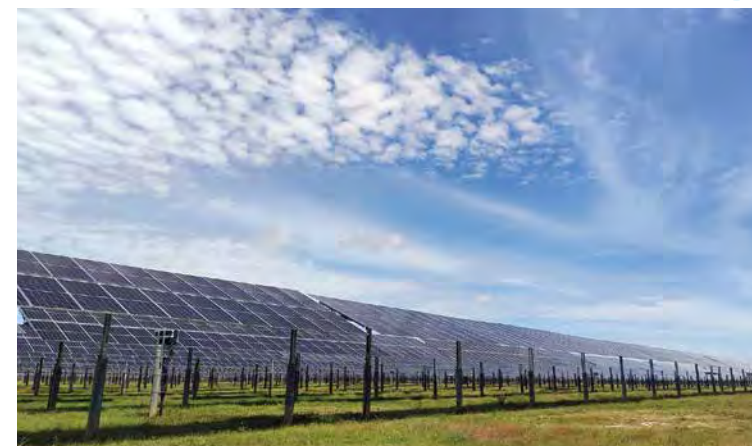
Visual 03: Coara Marang's solar site in Terengganu
